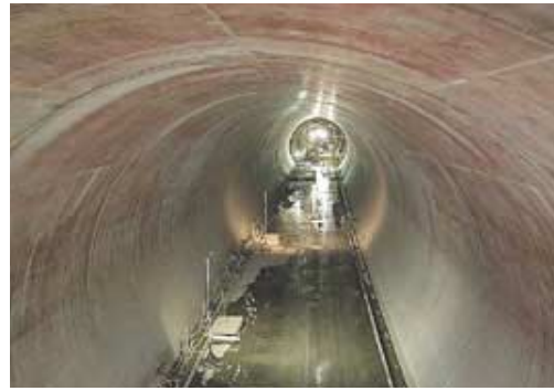
Figure 2: The interior of the North Down's Tunnel, which is coated in fibre-enhanced concrete.
