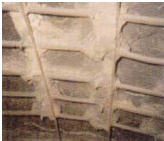
Figure 1: Fire spalling of concrete lining in the Channel Tunnel 1996. 3
